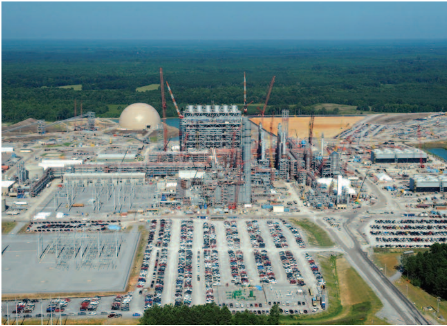
Kemper County Project (EPA's "Kill Coal" Plan). This project is one of four demonstration coal-fired CO 2 sequestration plants under construction. Owned by Southern Company, the company received a $270 million grant from the Department of Energy. Southern Company has issued a statement saying the Kemper technology "cannot be consistently replicated on a national scale." The EPA claims it can be commercially built and operated competitively. Who do you believe? Photo taken in September 2013. Completion expected in late 2014. SOURCE: WIKIMEDIA COMMONS
