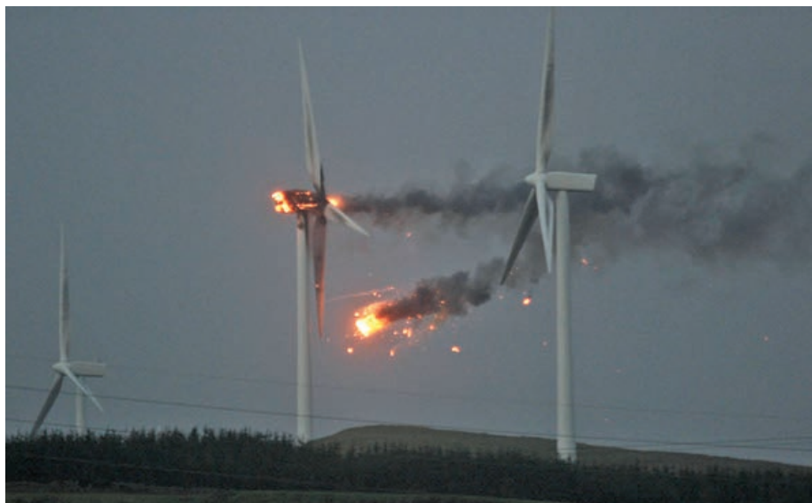
Turbine failure in high winds, North Ayrshire, Scotland. The rate of failure of wind turbines and towers far exceeds expectations, requiring more frequent replacement, shorter life expectancies, and higher costs. SOURCE: Stuart McMahon, used with permission.
